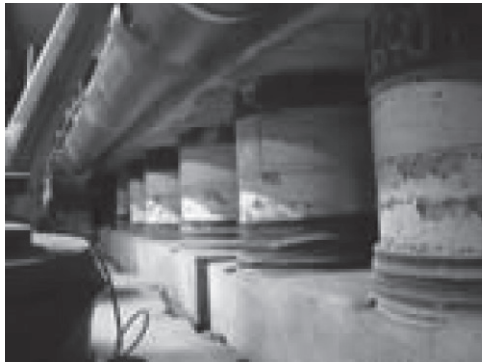
(a) Highly deformable concrete slots (Solexperts HDC®) in Chienberg tunnel (Jura Mountains).
